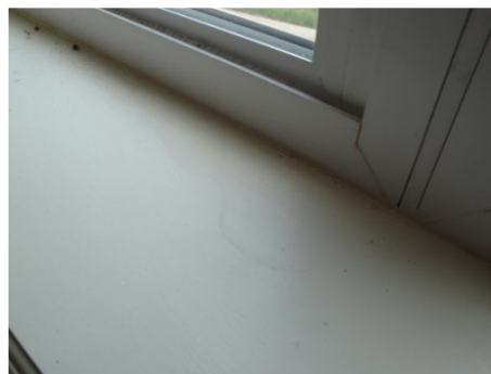
Figure 10: Interior of a north window (inside of window in figure 9) had a moisture stain in the middle of the interior window sill.
