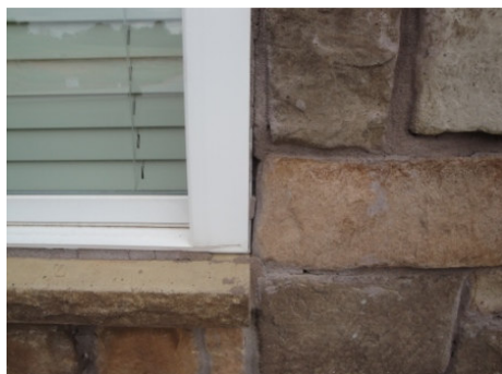
Figure 13: Window mortar missing from bottom right of window may be responsible for allowing moisture to enter the east bedroom.
