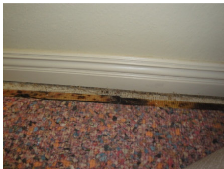
Figure 14: Area of floor beneath the missing mortar of the window from figure 13 was showing moisture stains and rusting nails.
