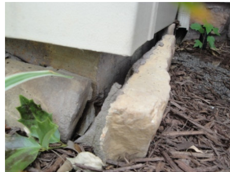
Figure 6: Siding rock loose from side of slab.
