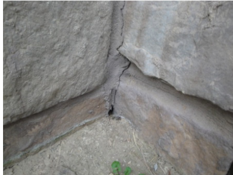
Figure 1: A hole in a corner of the stone siding to be filled/sealed.
