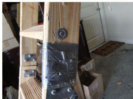
Figure 7: Duct taped attic ladder.
