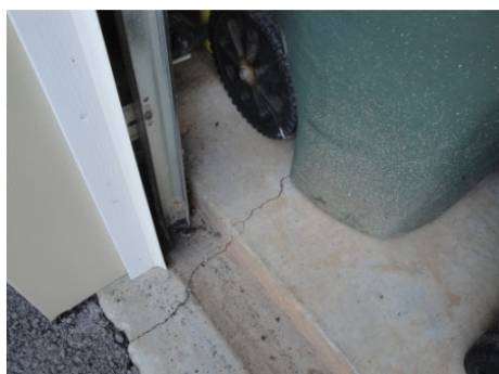
Figure 17: The beginning of a concrete floor crack in the garage could not be further evaluated due to current tenants' stored items.
