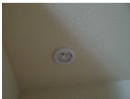
Figure 16: Missing smoke detector in master bedroom.
