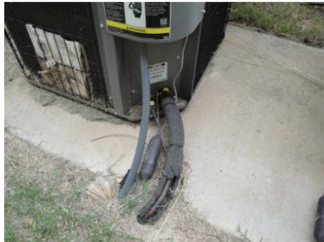
Figure 3: Insulation of refrigerant lines was in need of replacement.
