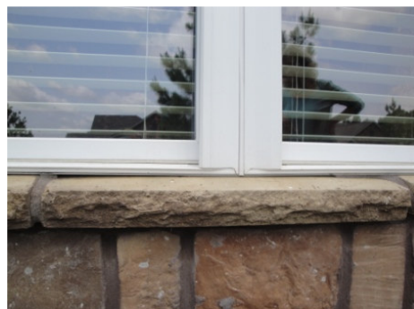
Figure 9: Another unlevel sill where the window sash bottom was not sealed properly.
