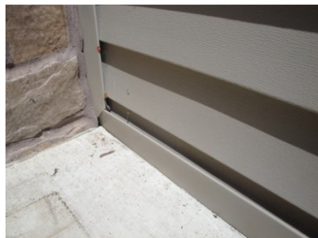
Figure 11: Hole at floor corner of the front entry and wall/floor connection could possibly be responsible for allowing moisture into the NE room.
