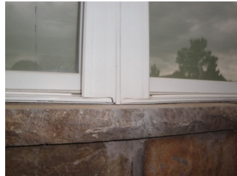
Figure 4: Window sash took form of unlevel sill.
