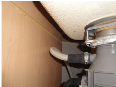
Figure 1: Bring the dishwashing machine drain line up to where it is higher than the bottom of the sink basin.
