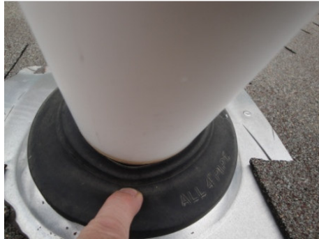
Figure 9: Rubber boot of a north plumbing vent could have pushed down during heavy rains and allowed water to travel downwards.
