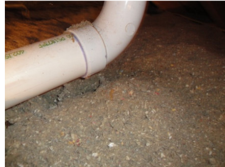
Figure 10: Moisture beneath the plumbing vent viewed from the attic.
