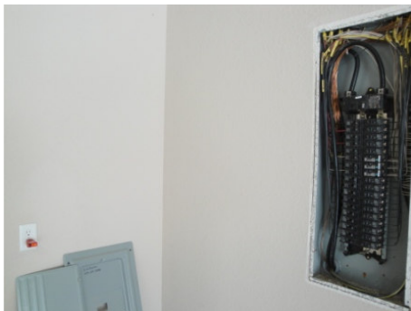
Figure 5: The electrical outlet in the NW corner of the garage did not appear to be GFCI protected.
