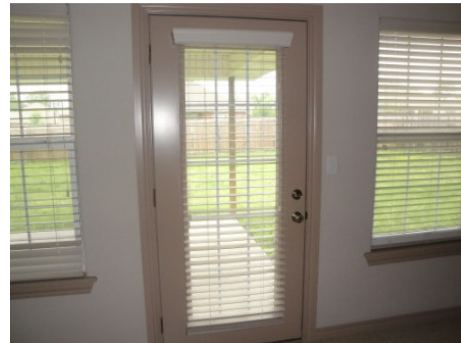
Figure 8: Windows within 2 feet from the back exterior door did not appear to be safety tempered glass.
