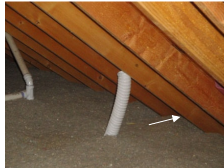
Figure 2: Bathroom exhaust fan extension could be taken off its nail and laid down toward the soffit venting of the eave.
