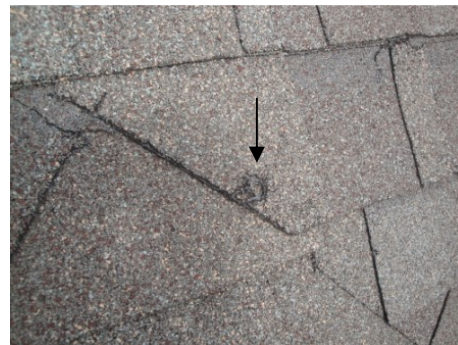
Figure 4: Several small holes were noted in the shingles.
