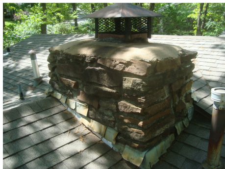
Figure 9: Chimney chase flashing in need of repair.
