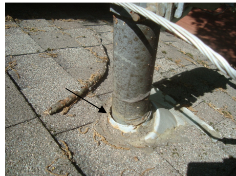
Figure 6: Gap to seal at the base of the electrical masthead.
