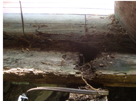
Figure 2: Some areas under the seats were rotted and in need of repair.
