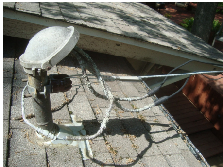
Figure 5: Electrical service wires covering was flaking/unraveling.
