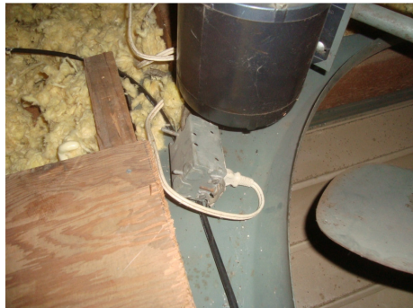
Figure 3: Loose electrical outlet in the attic.
