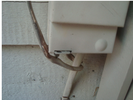
Figure 19: Wire insulation wearing where it wrapped around this disconnect box of A/C compressor #1.
