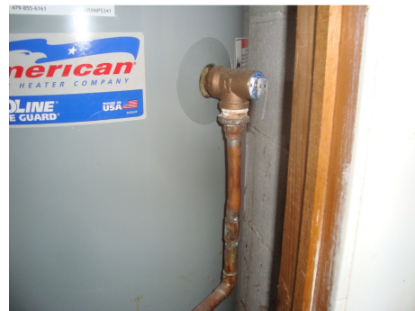
Figure 18: Water heater #1 with a necked down temperature/pressure valve extension.
