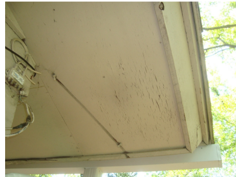
Figure 8: Soffit with peeling paint. This type of peeling may indicate that moisture is getting on the backside of the soffit.
