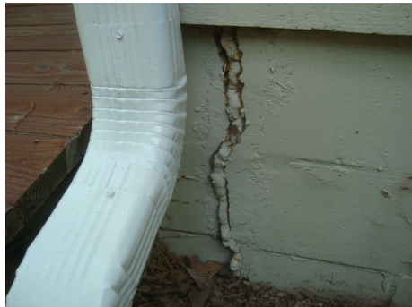
Figure 13: Settlement/shifting of the SW corner of the original foundation (outside master bedroom).
