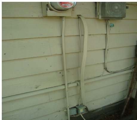
Figure 11: Large energized electrical lines run outside the siding and not run in conduit.
