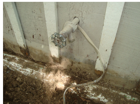
Figure 12: Electrical line sharing a wall penetration on the east exterior. The electrical wire was tested and the line was not energized at that time it was tested.
