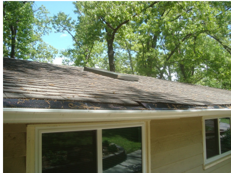
Figure 15: Dip in roof line and attached gutter.
