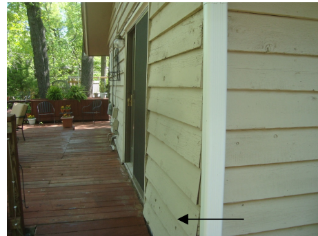
Figure 14: Wall appeared to be kicked out towards the bottom.
