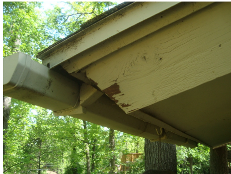
Figure 7: Facia with peeling paint.
