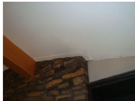
Figure 10: Area of moisture penetration at ceiling and fireplace connection.
