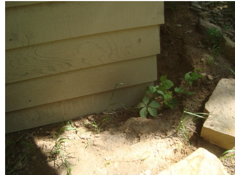
Figure 16: Wood siding in contact with the soil.
